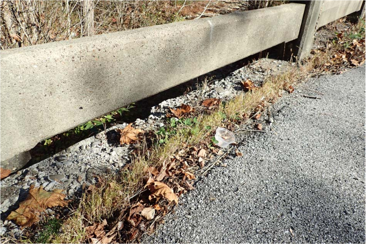
Moderate scaling/spalling along the top of the downstream curb near abutment 1.
