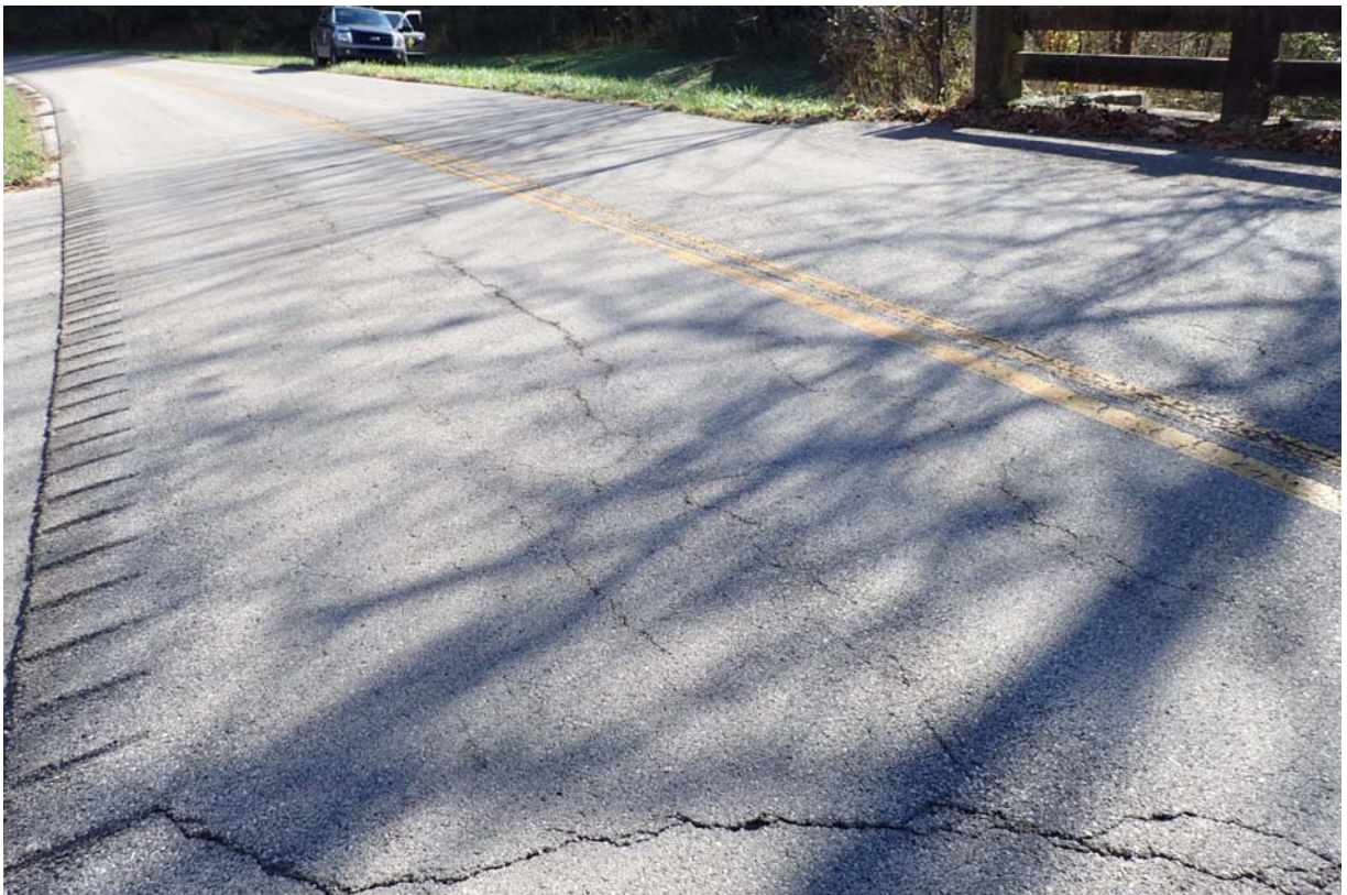
Typical view of the asphalt wearing surface. Notice the moderate sized transverse cracking at the end of the bridge and the moderate sized longitudinal cracking in the driving lanes.
