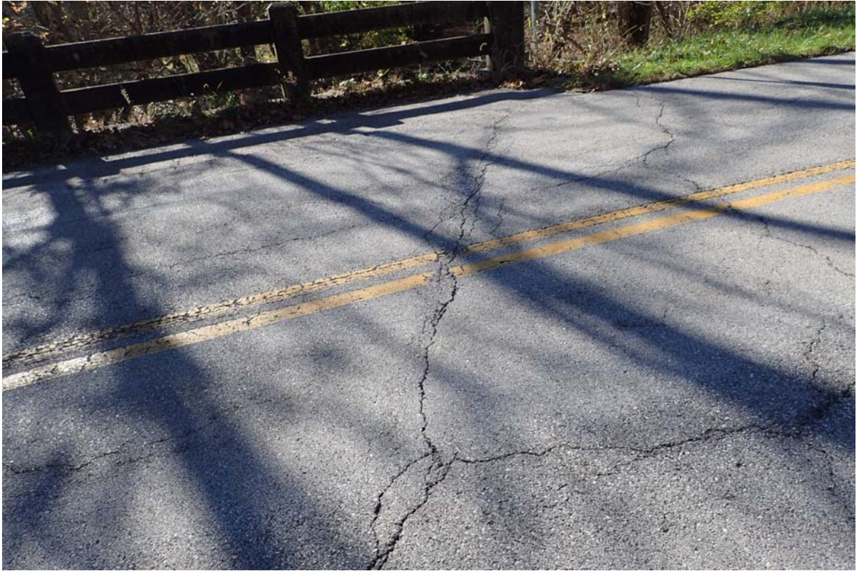
Typical view of moderate sized transverse cracking in the asphalt wearing surface over abutment 1.
