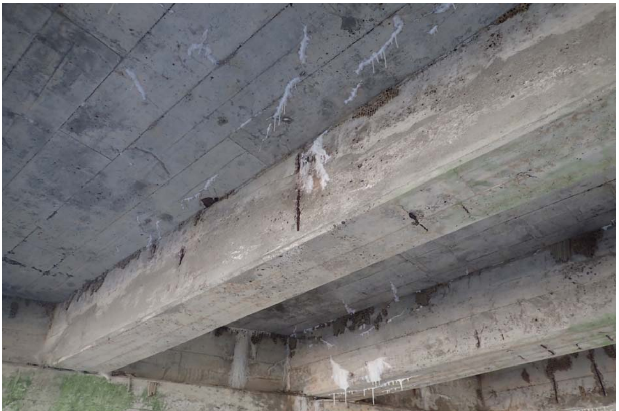
View of beam 6 near abutment 2. Notice the shallow spalls with exposed steel.
