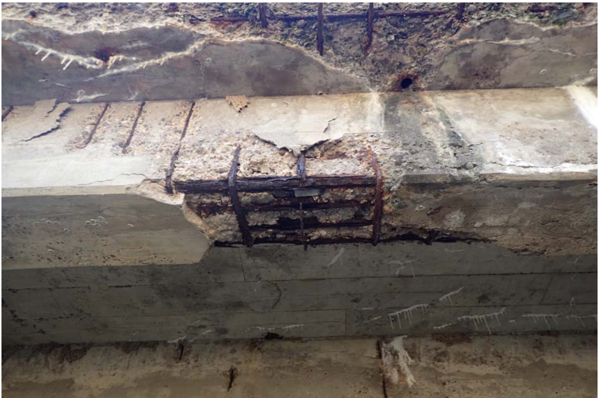
Heavy spalling with exposed steel in the downstream exterior girder below the deck drain near abutment 2. Notice the heavy corrosion of the steel reinforcement.
