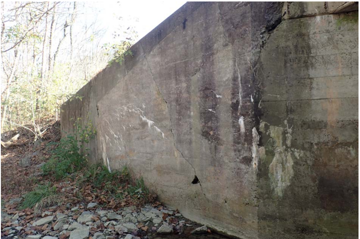
View of abutment 2s downstream wingwall. There are 2 full height vertical cracks and an area of minor sized cracking with efflorescence of heavy intensity.
