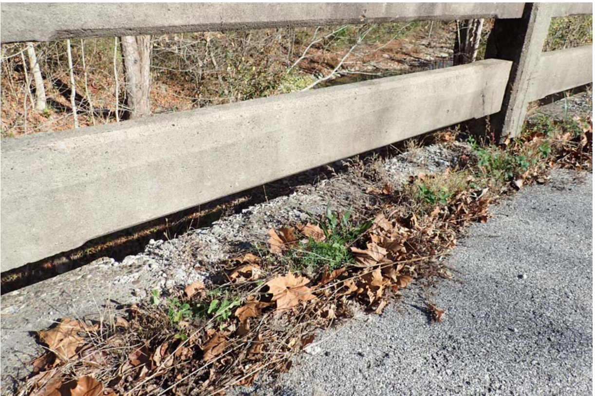
Moderate scaling/spalling along the top of the downstream curb near midspan.
