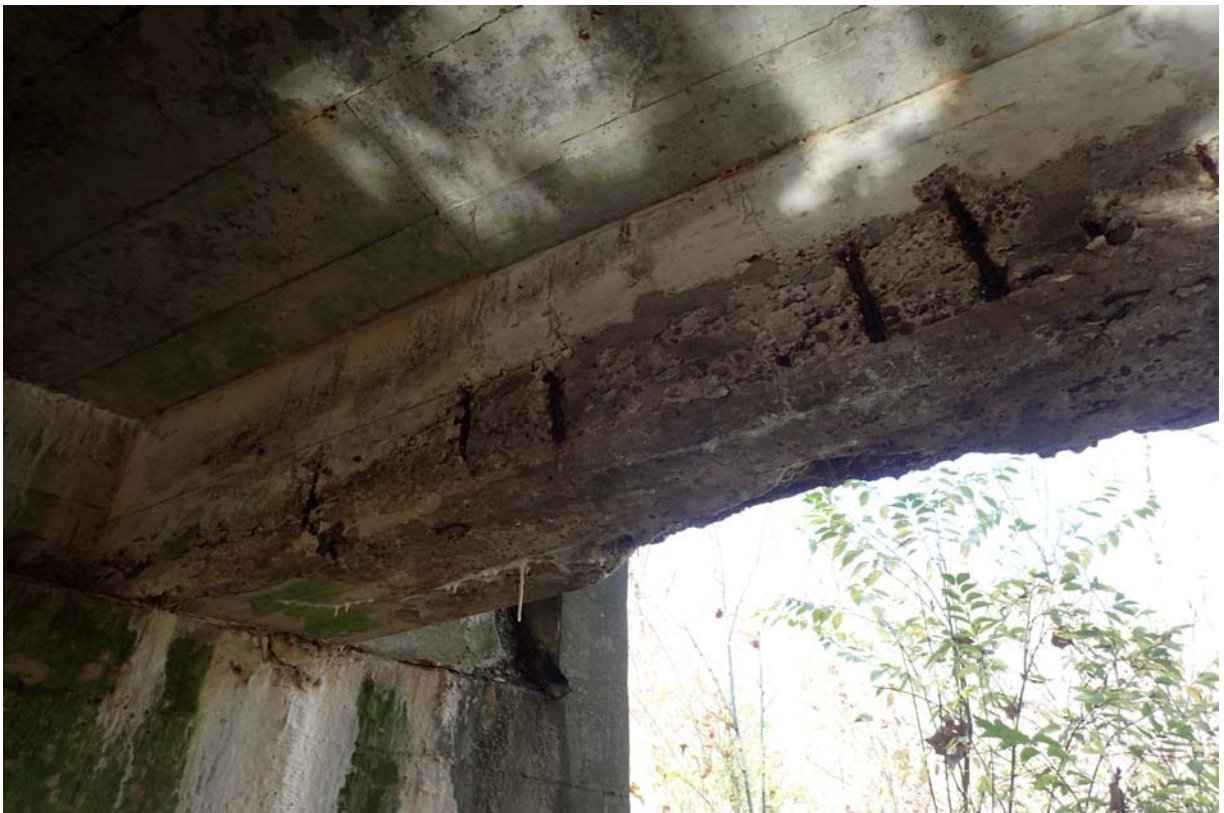
Several shallow spalls with exposed steel along the interior face of the downstream beam near abutment 1.
