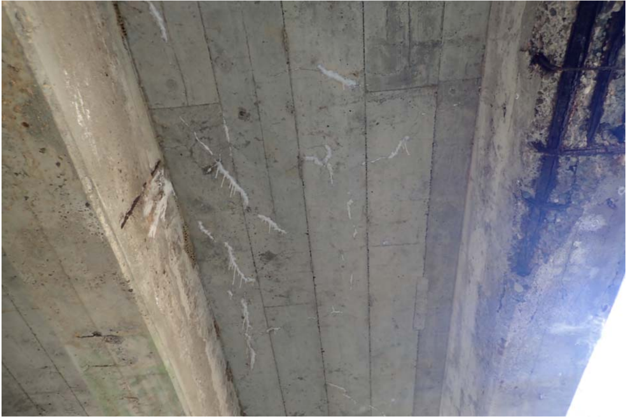
View of minor cracking with efflorescence in the deck underside between beams 6 and 7 from upstream.
