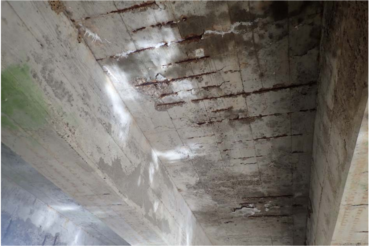
Shallow spalling with exposed steel in the deck underside between beams 5 and 6 from upstream. Photo taken from abutment 1 looking toward midspan.
