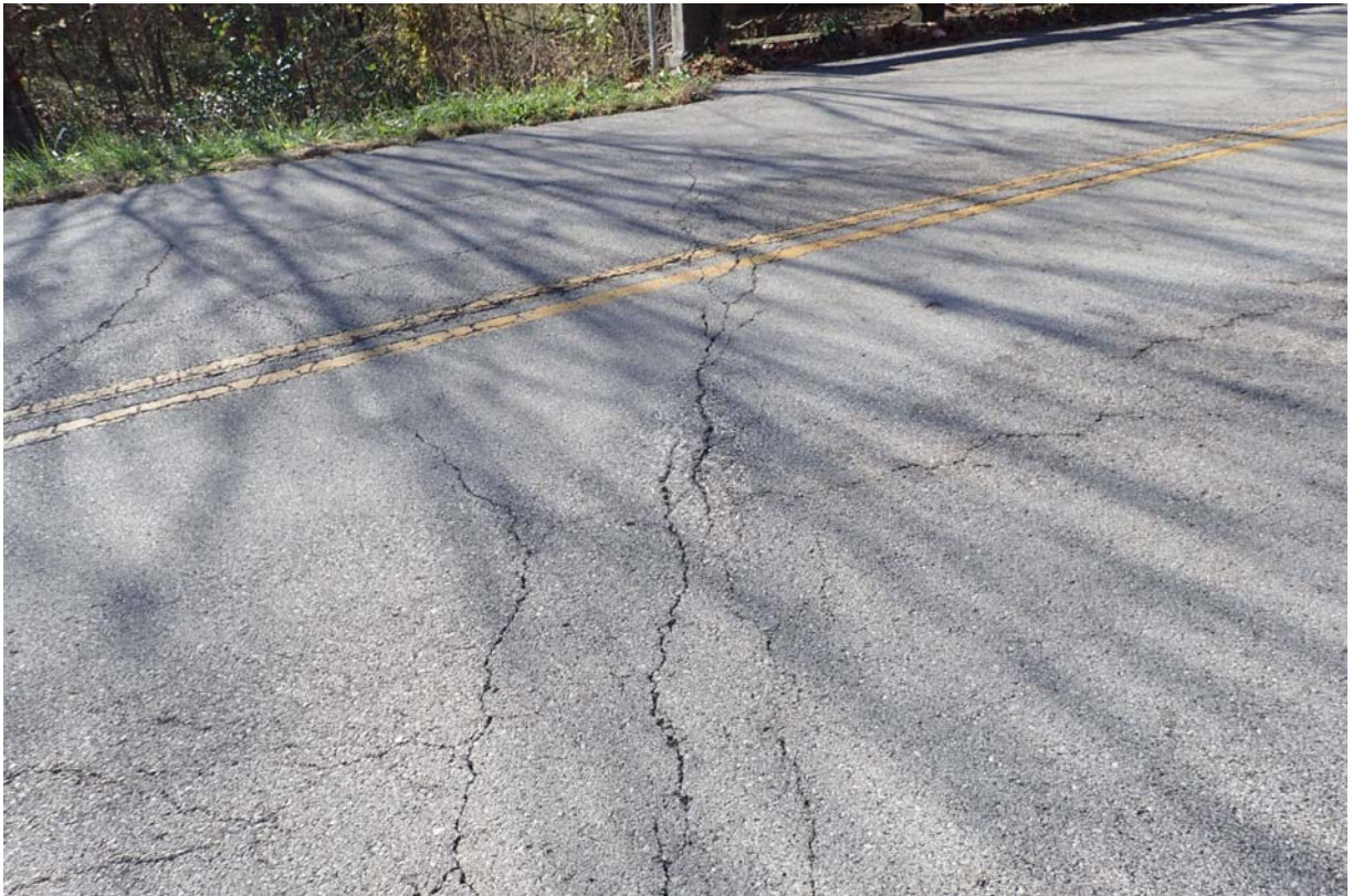
Typical view of moderate sized transverse cracking in the asphalt wearing surface over abutment 2.
