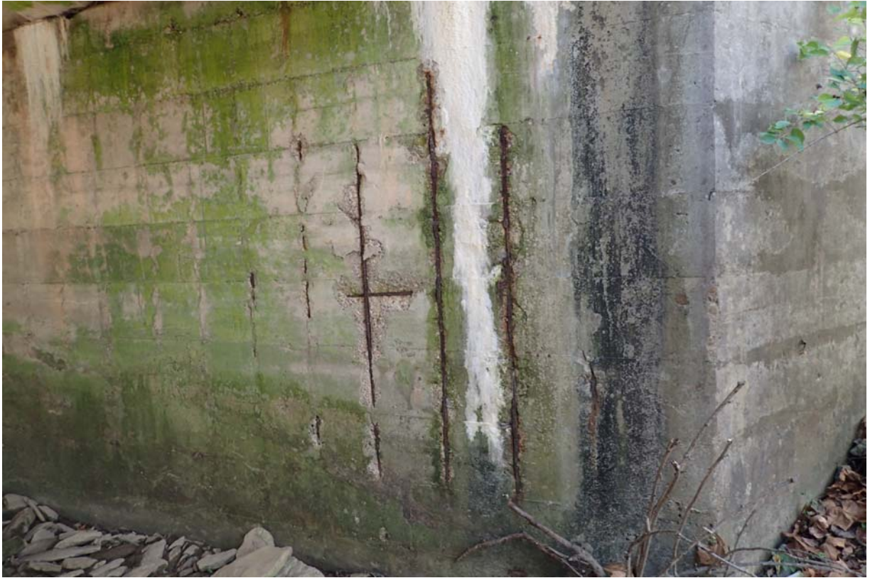
Shallow spalling with exposed steel at the downstream end of abutment 1.
