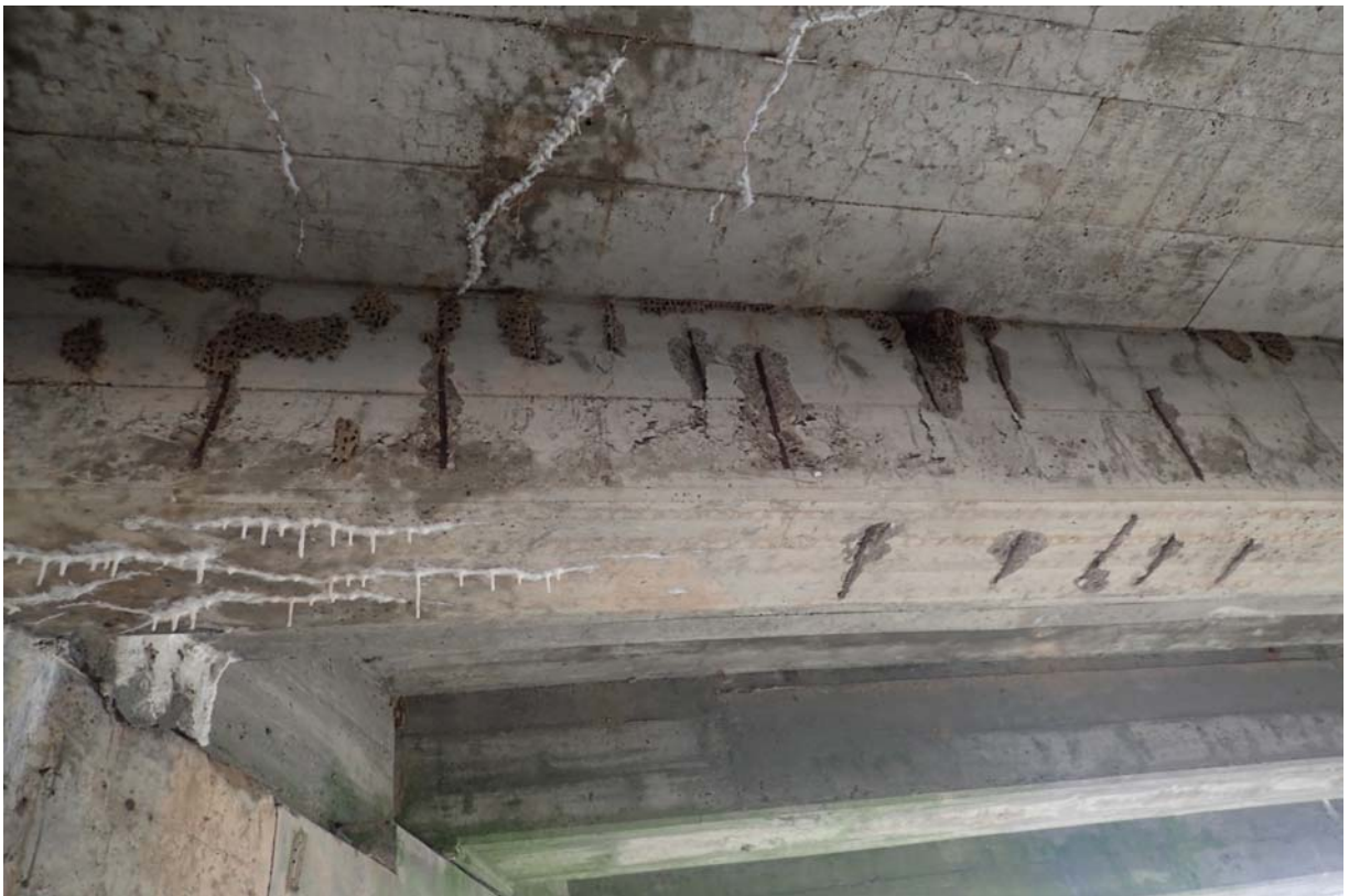
View of the downstream face of beam 4 from upstream near abutment 2. Notice the several shallow spalls with exposed steel.
