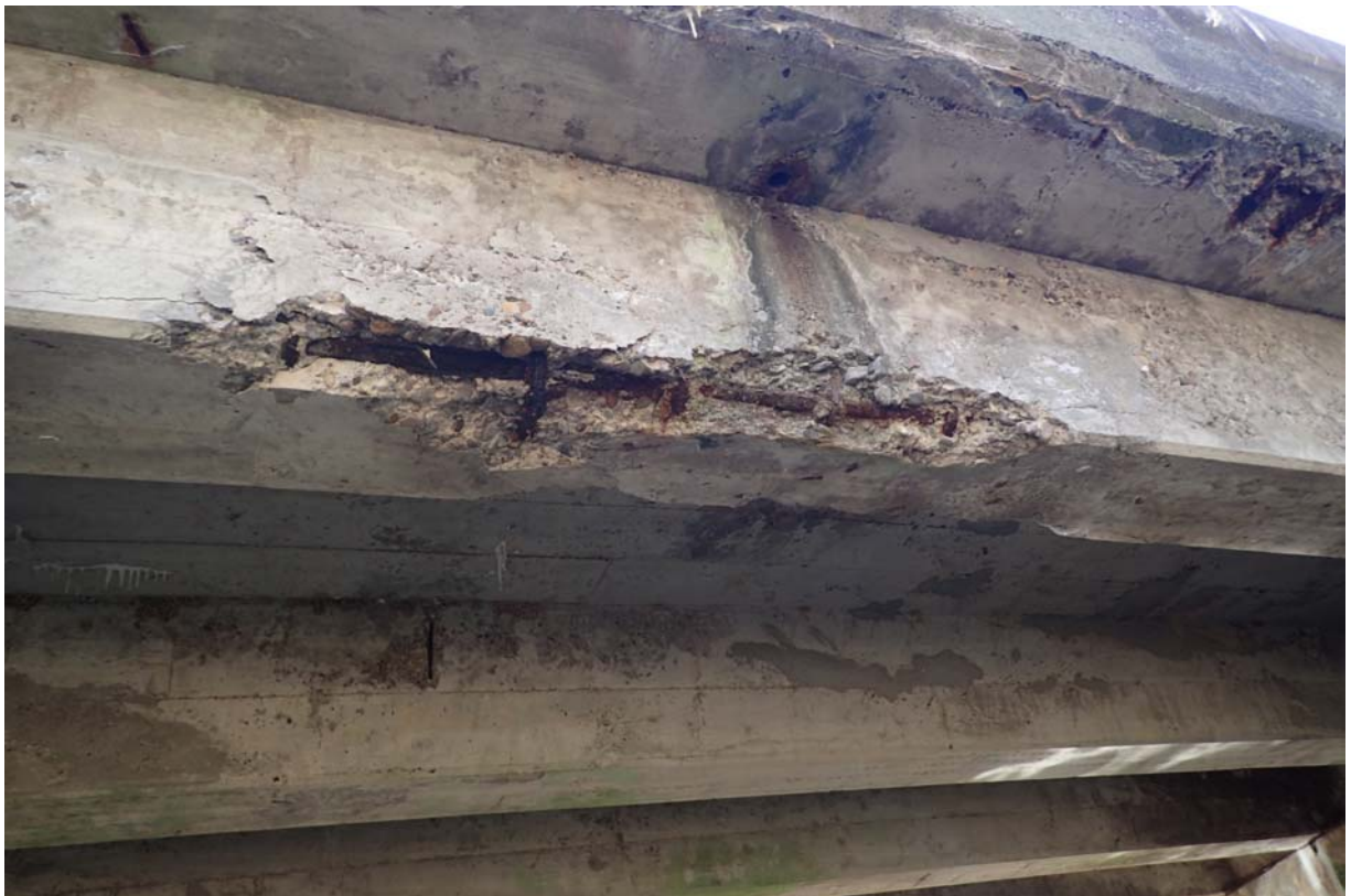
Heavy spalling with exposed steel in the downstream exterior girder below the deck drain near midspan. Notice the heavy corrosion of the steel reinforcement.
