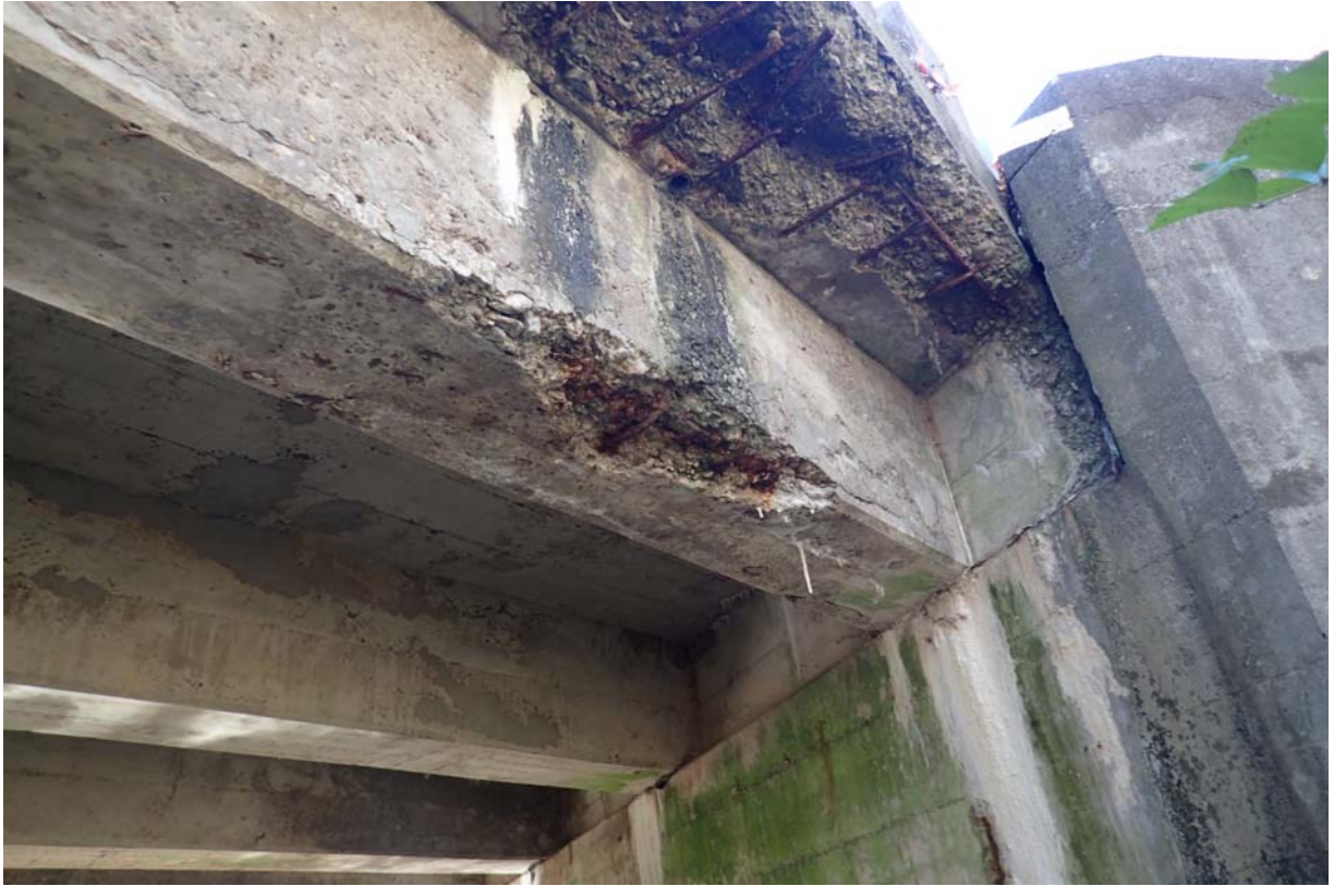
Heavy spalling with exposed steel in the downstream beam near abutment 1.
