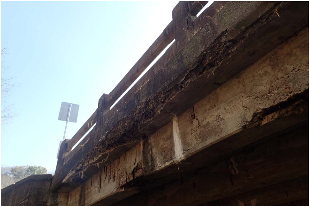
Heavy cracking and spalling in downstream deck overhang, extending from near abutment 2 to near midspan.
