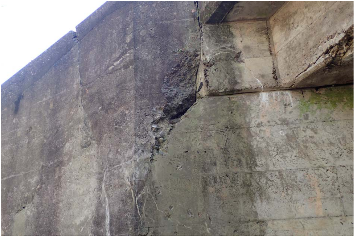
Fairly large deep spall in abutment 2 near the wingwall connection adjacent to the downstream end of the diaphragm
