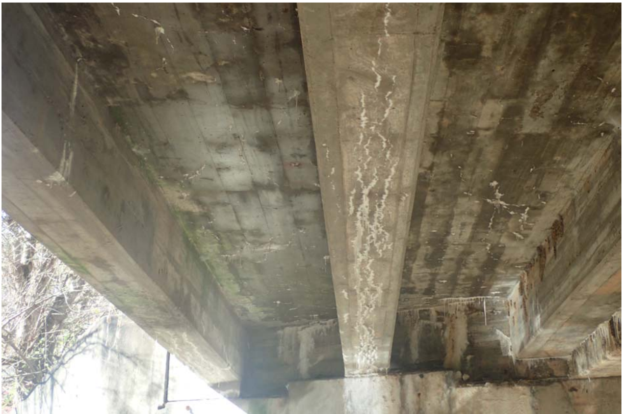
Typical view of beam 2 from upstream. Notice the heavy intensity of minor sized cracking.
