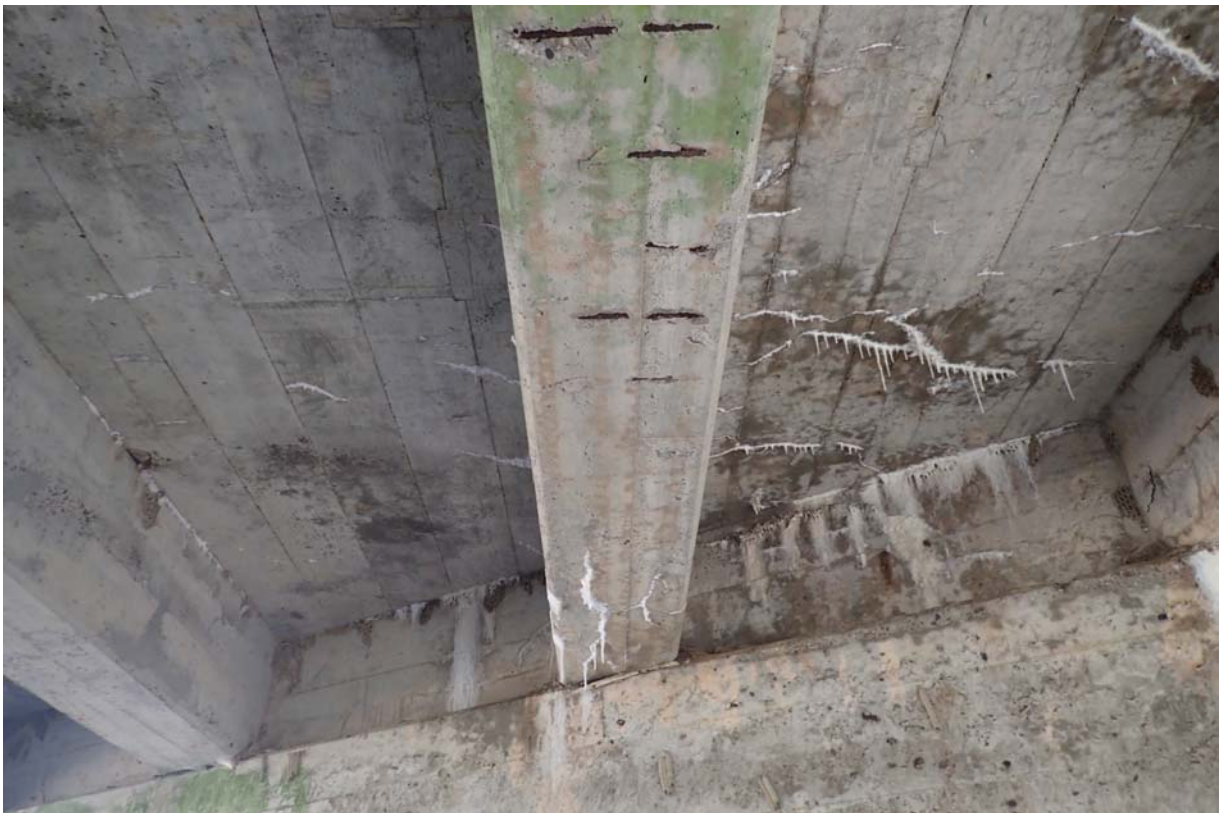
View of moderate intensity cracking with efflorescence and shallow spalling with exposed steel in the underside of beam 5 near abutment 2.
