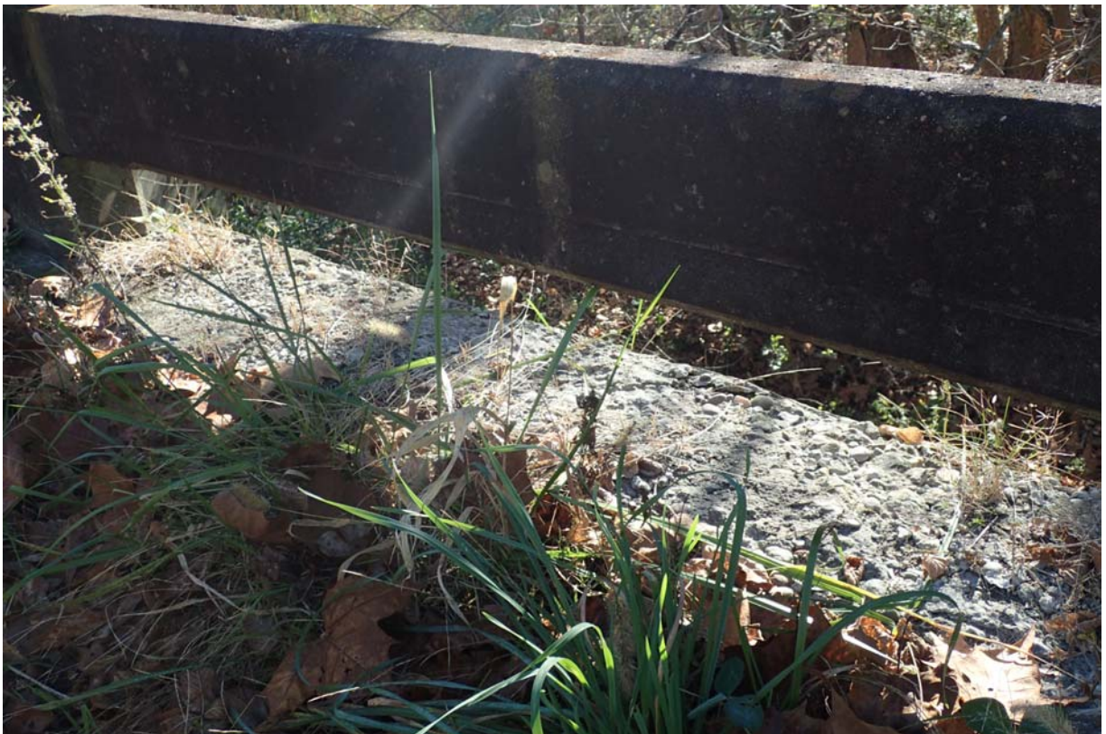
Moderate scaling/spalling along the top of the upstream curb near midlength.
