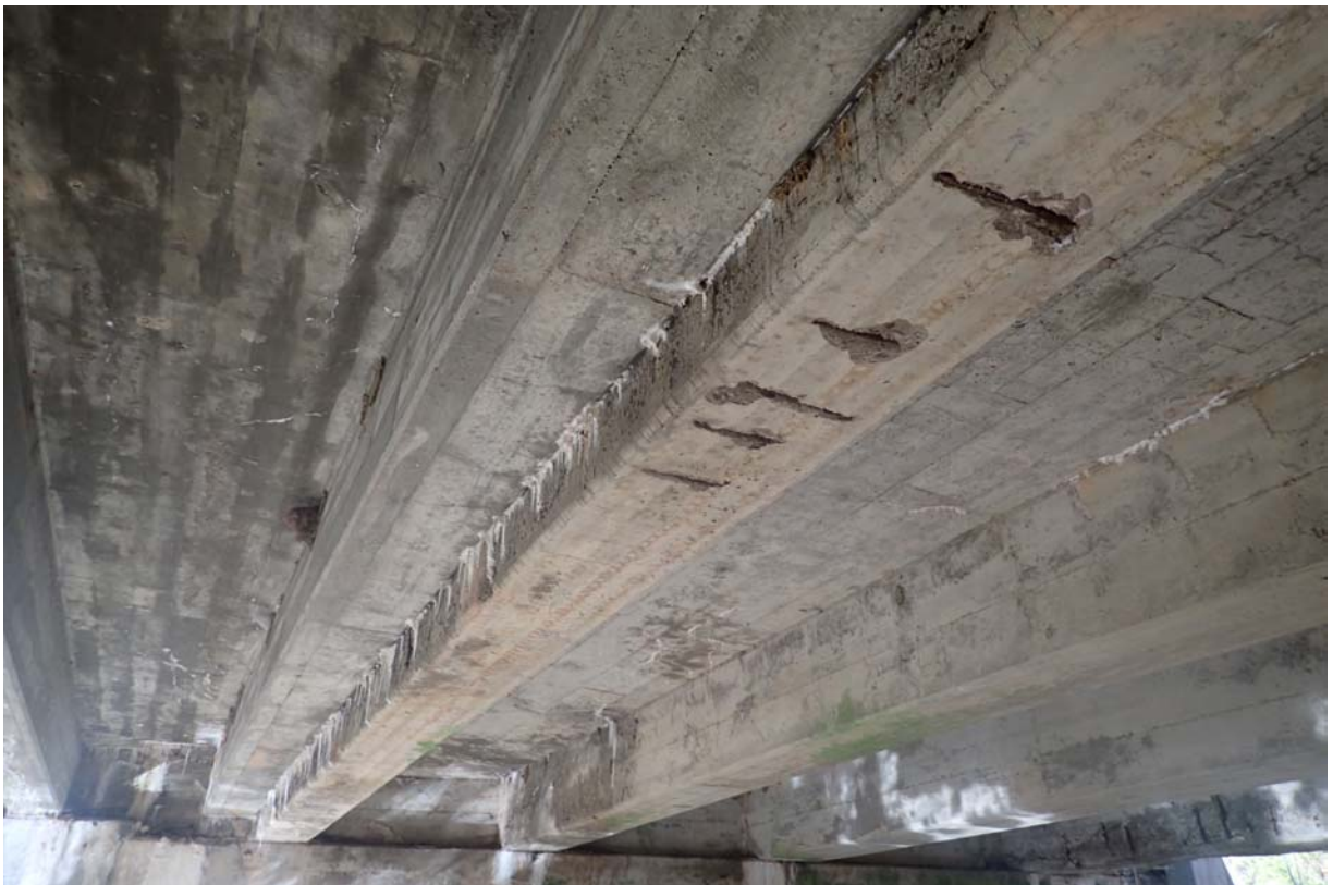
Typical view of beams 3 and 4 from upstream. Notice the several shallow spalls with exposed steel in the underside of beam 4 from upstream near abutment 2.
