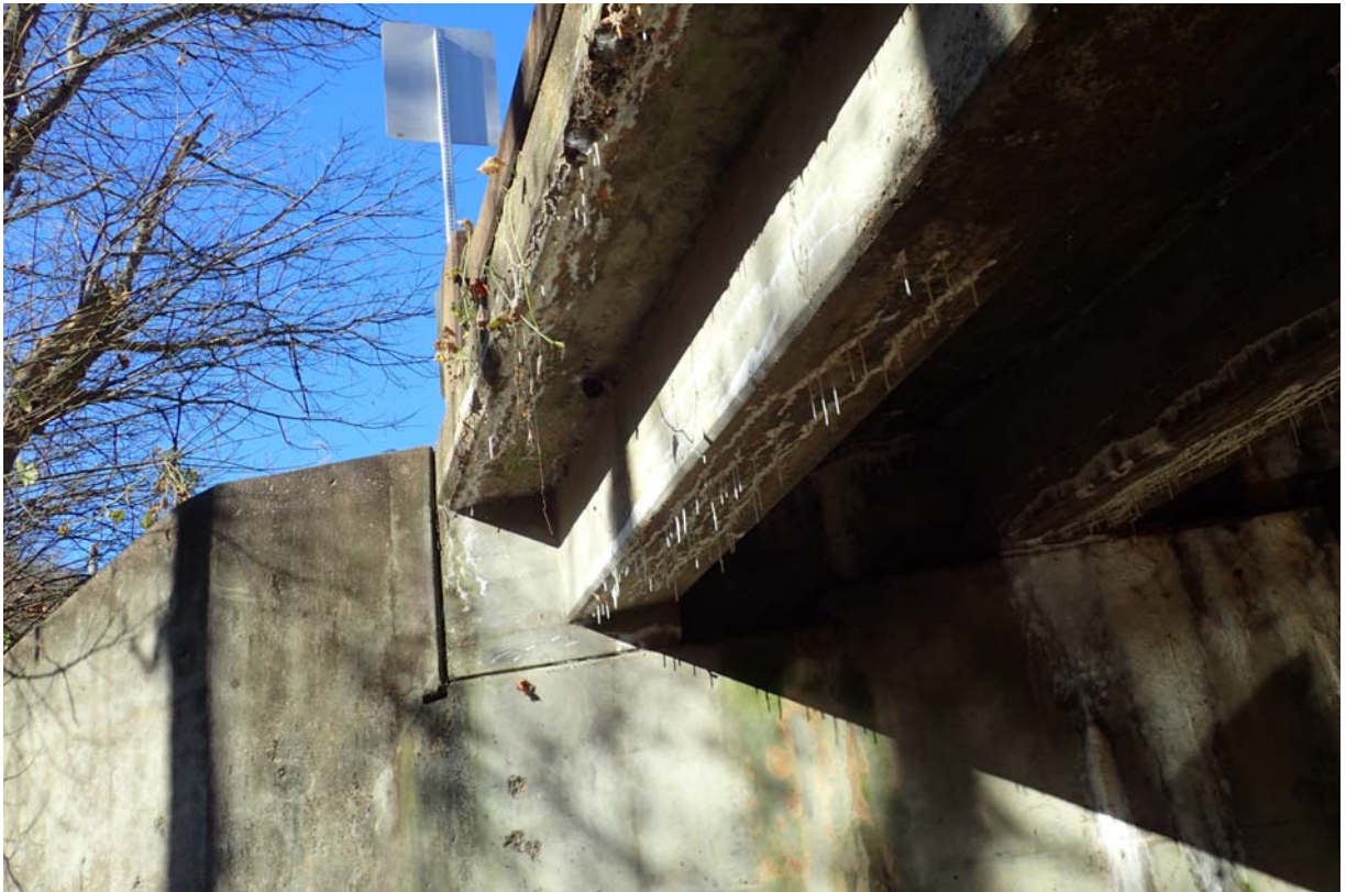
Typical view of minor sized cracking with efflorescence of heavy intensity in the upstream beam (beam 1) near abutment 1.
