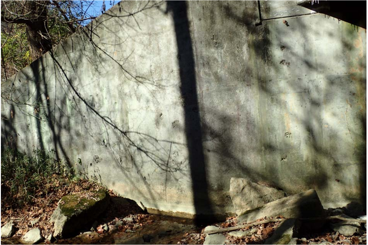
Several minor sized spalls at the upstream end of abutment 1.
