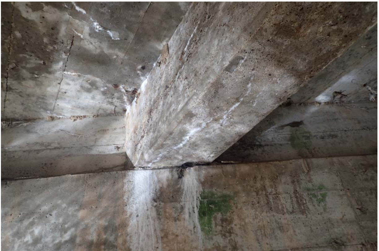
Moderate intensity of minor sized cracking with efflorescence in beam 5 at abutment 1.
