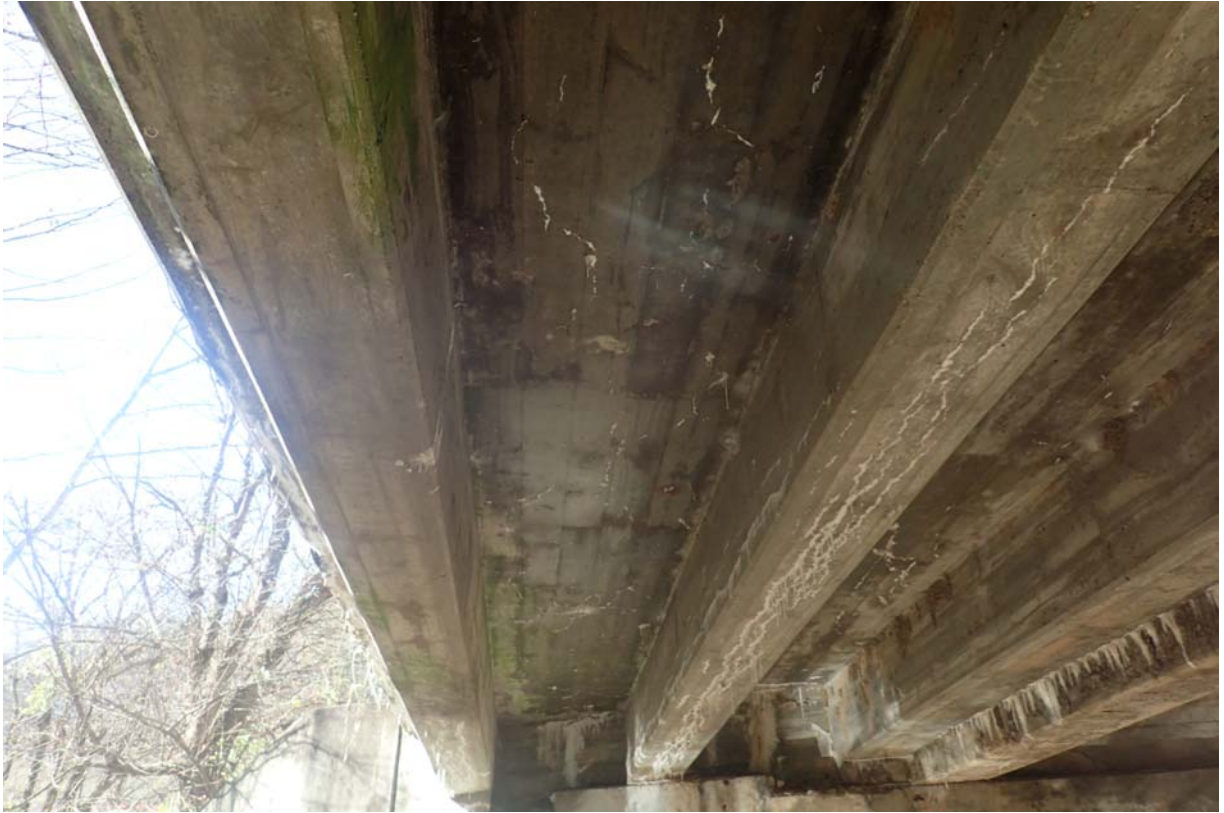
View of dark discoloration with scattered minor sized cracks with efflorescence in the deck underside between beams 1 and 2 from upstream.
