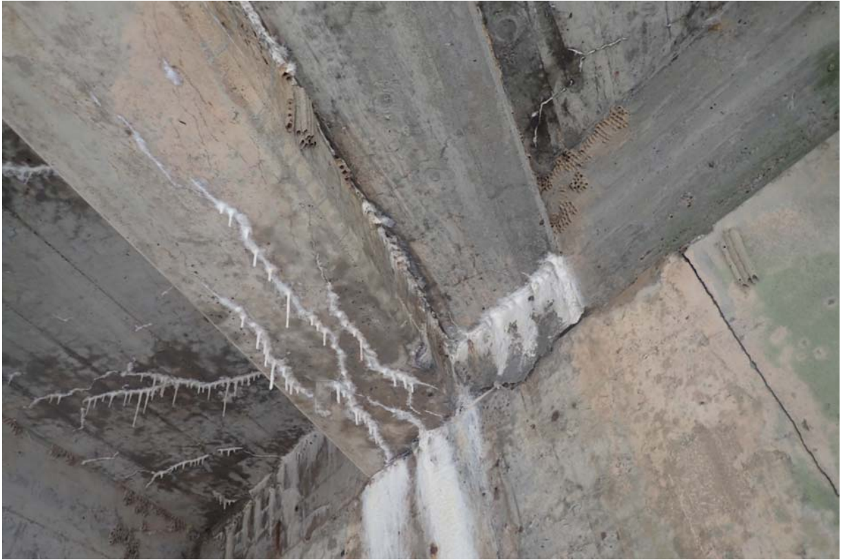
Heavy intensity of minor sized cracking with efflorescence at the end of beam 4 at abutment 2.
