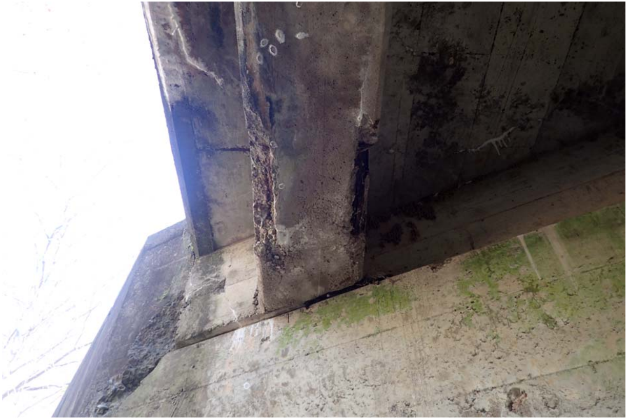
Moderate spalling with exposed steel in the downstream girder at abutment 2.
