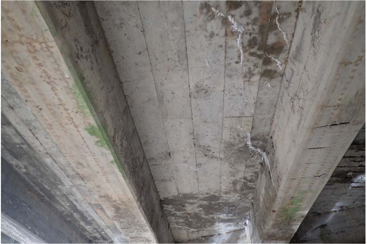
Typical view of the deck underside between beams 4 and 5 from upstream. Photo taken from midspan looking toward abutment 1.
