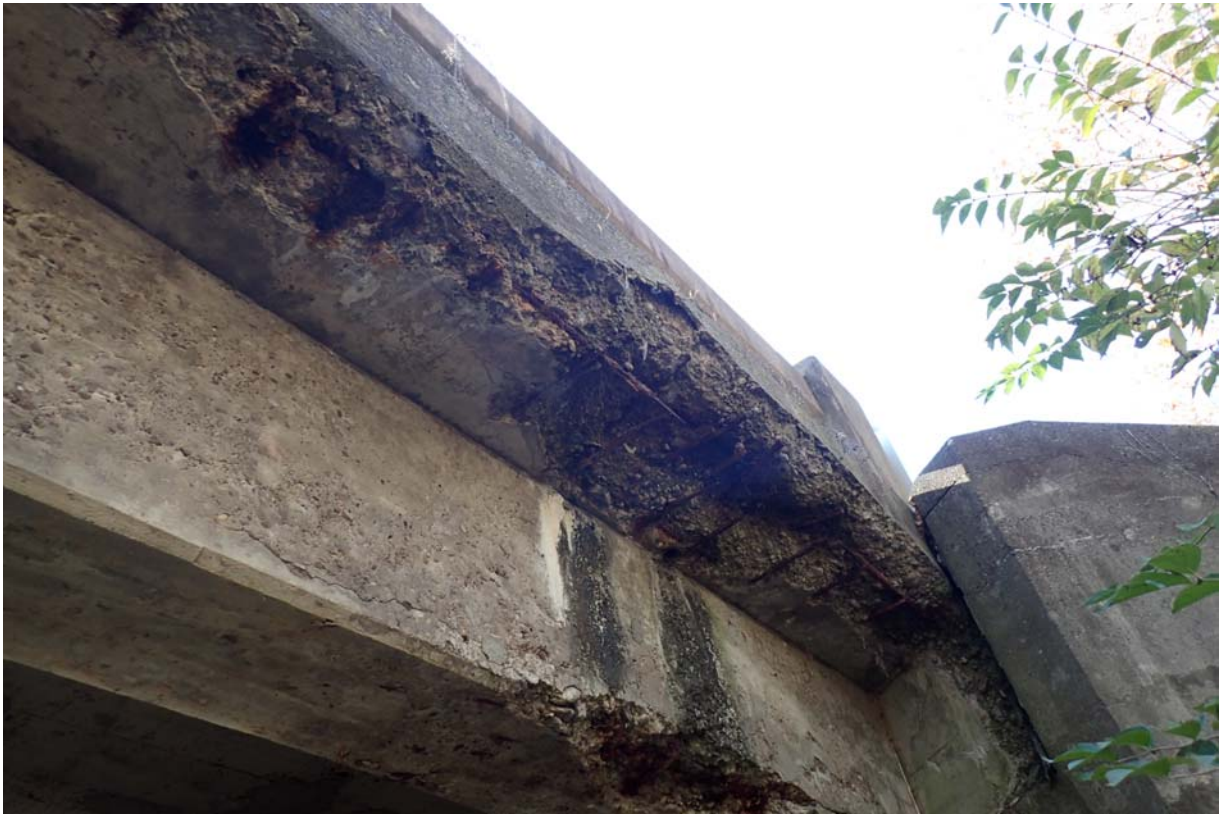
Heavy spalling with exposed steel in the downstream deck overhang near abutment 1.
