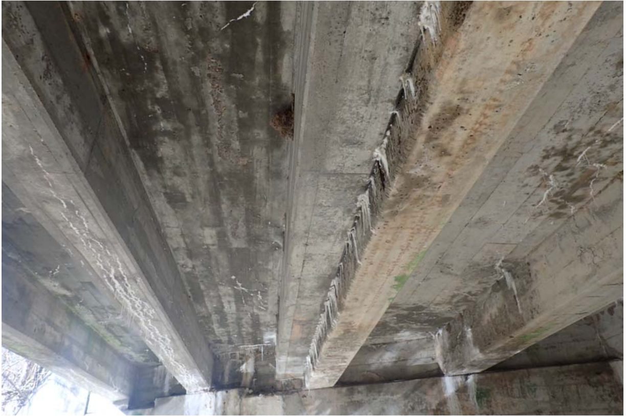
View of dark discoloration with scattered minor sized cracks with efflorescence in the deck underside between beams 2 and 3 from upstream.
