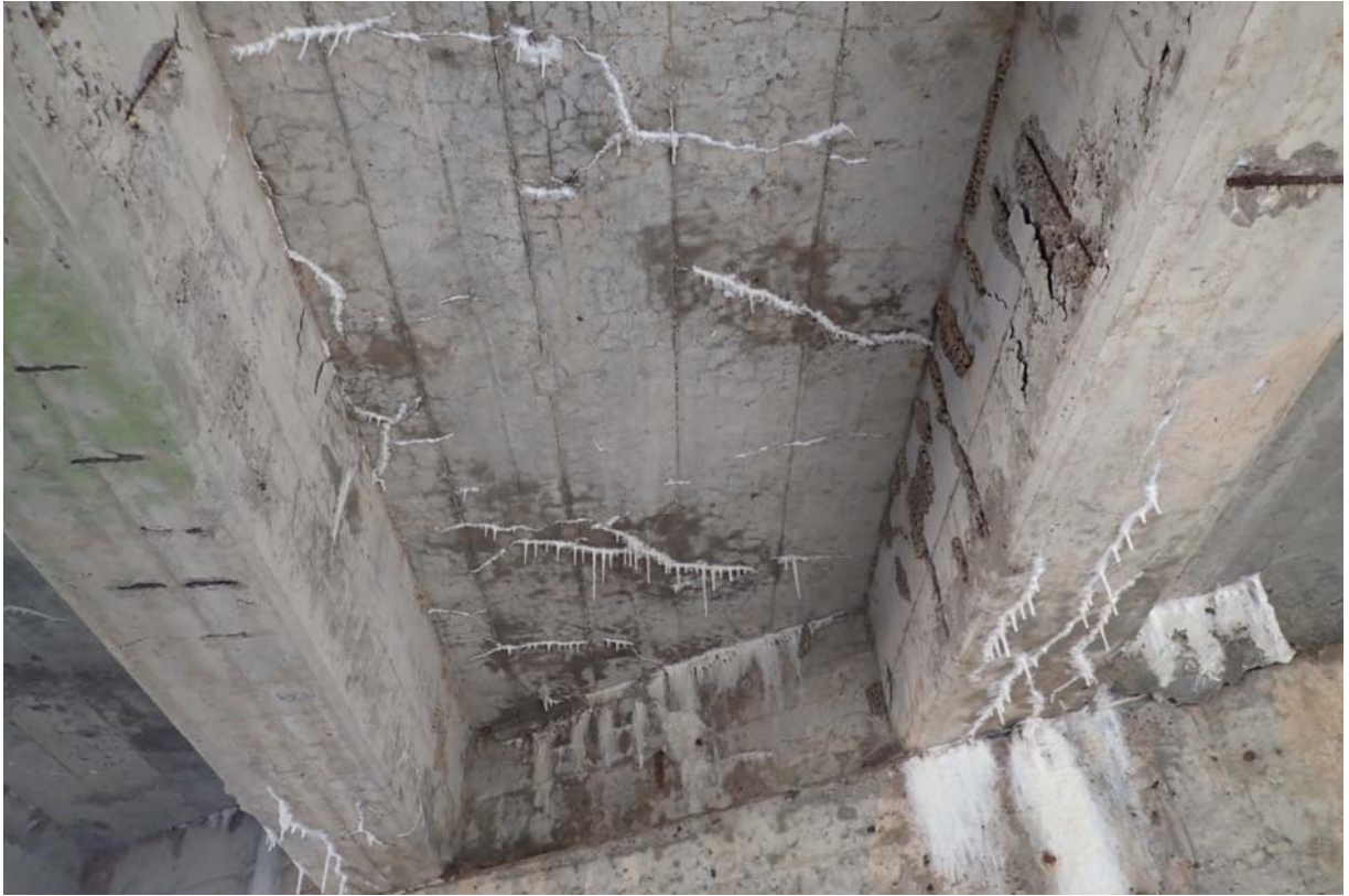
View of the deck underside with moderate to heavy intensity of cracking with efflorescence and discoloration between beams 4 and 5 from upstream near abutment 2.
