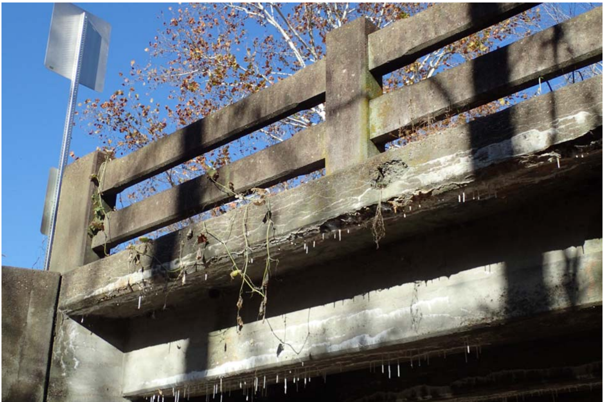
Heavy intensity of minor sized cracking with efflorescence and areas of moderate spalling in the upstream deck overhang near abutment 1.
