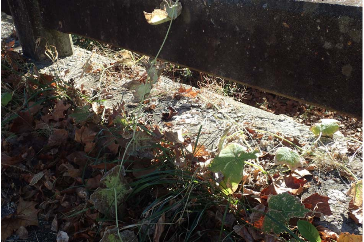
Moderate scaling/spalling along the top of the upstream curb near abutment 1.
