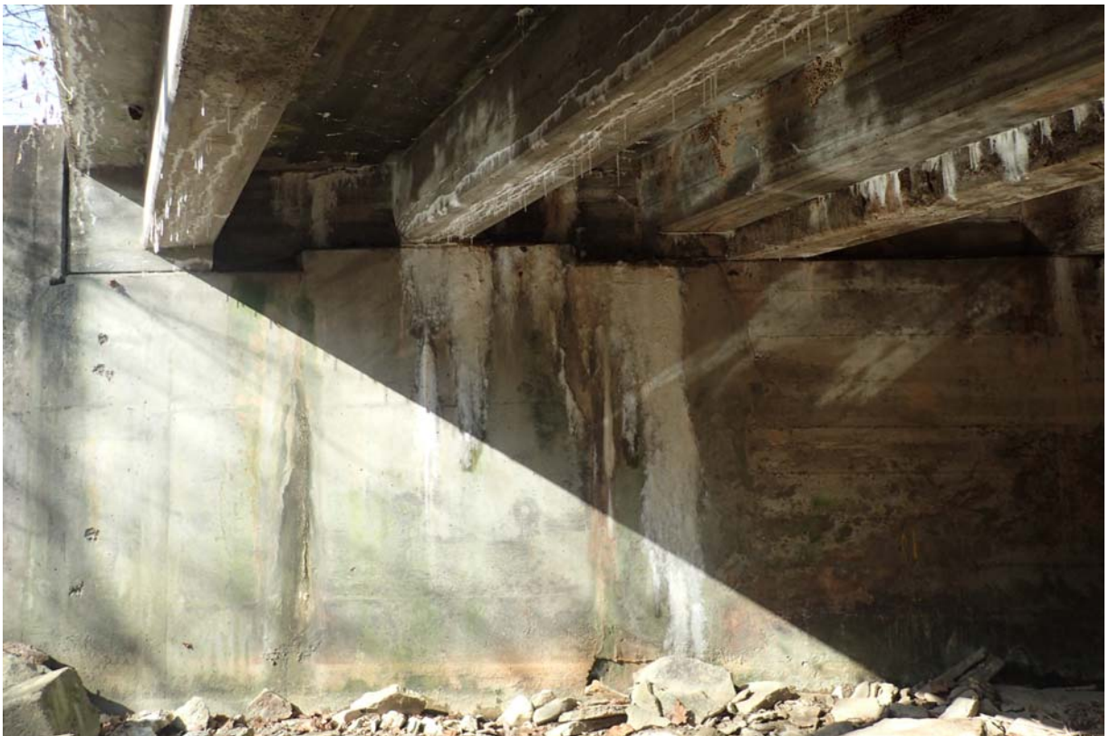
Heavy seepage at the seats of the upstream beams at abutment 1.
